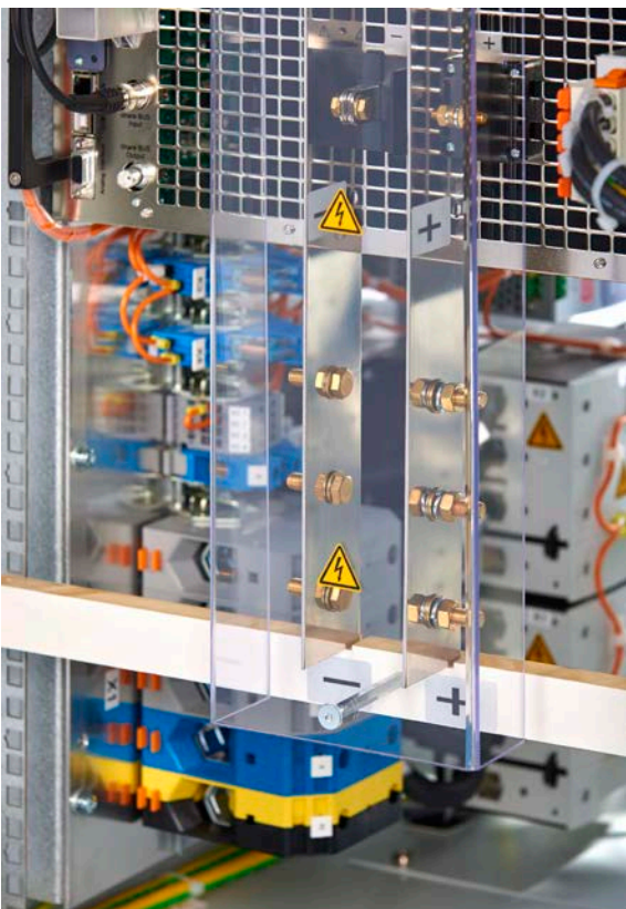
Closeup of the DC bus (24 U cabinet)
